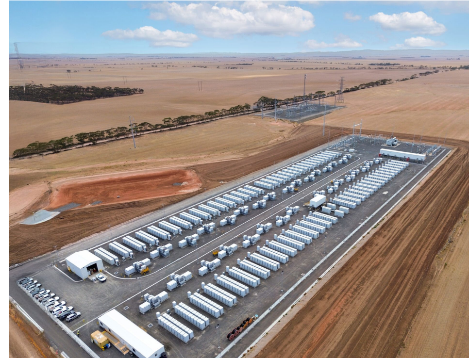
Blyth Battery - 238.50MW/447MWh – Connected 10 April 2025
